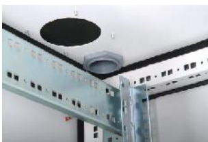
Sealed Cable Entry From Roof
